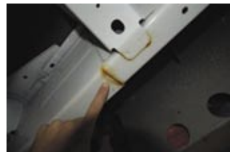
On this 2008 vehicle, there was already surface rust starting at the seams of this chassis section. Left untreated this would spread and could cause future problems
